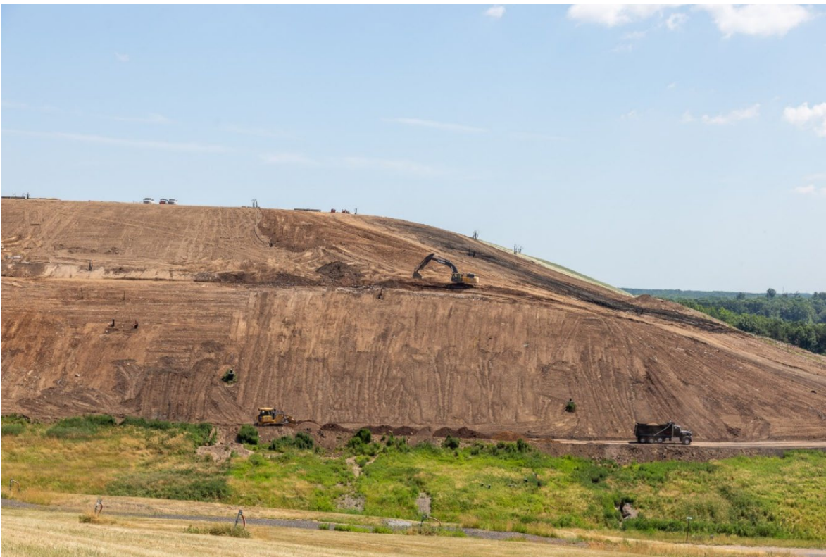
This photo shows the north side of the Phase III landfill before the installation began on the temporary cap.
