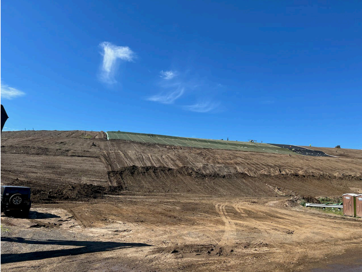
This photo shows the initial progress of the temporary cap installation, which is anticipated to be completed by August 15th, weather permitting.
